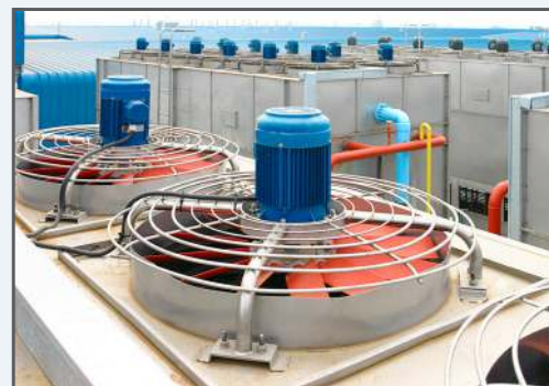
Fans and water pumps
