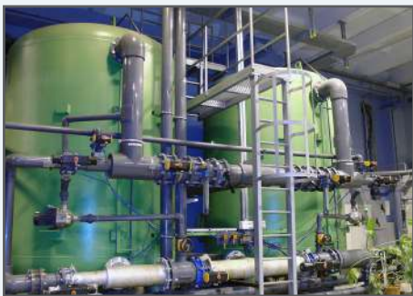
Environmental protection equipment
